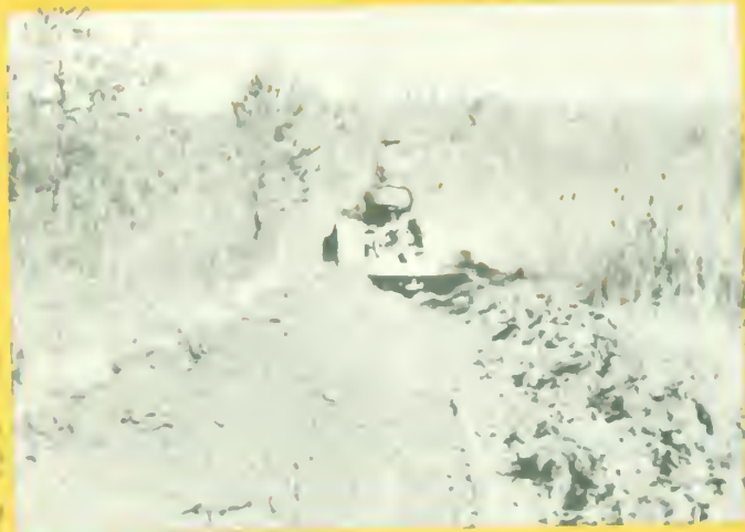
Light tractor-and-plow units construct effective firebreaks in a minimum of time in Piedmont and North Georgia.
